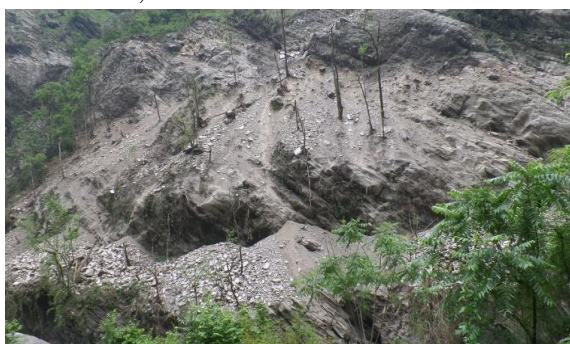
Figure 5-17: Deposition of demolition wastes produced during road construction, into the Budigandaki river
